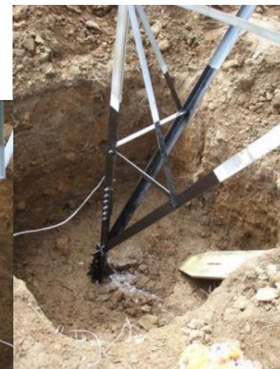
Pylons of ICE (Costa Rica)
