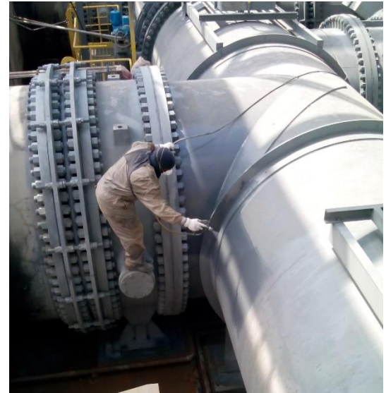
SAUDI ELECTRICITY COMPANY INTAKE VALVES AND PIPES
