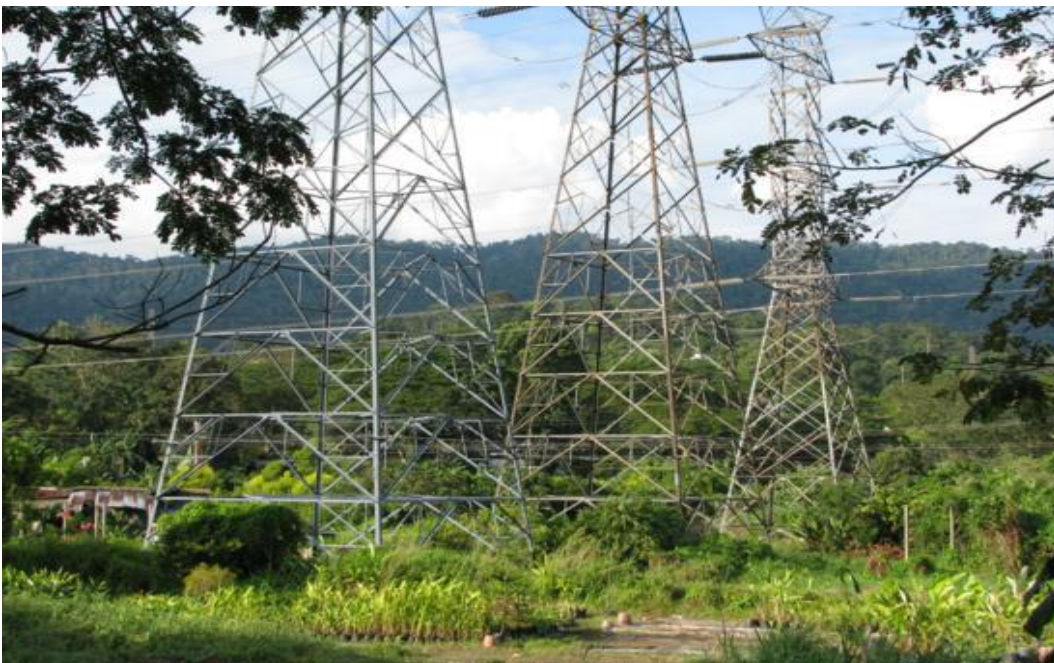
Left: pylon protected by ZINGA Right: 2 rusty towers not yet protected
